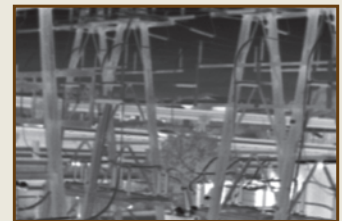
Medium-range plant surveillance
